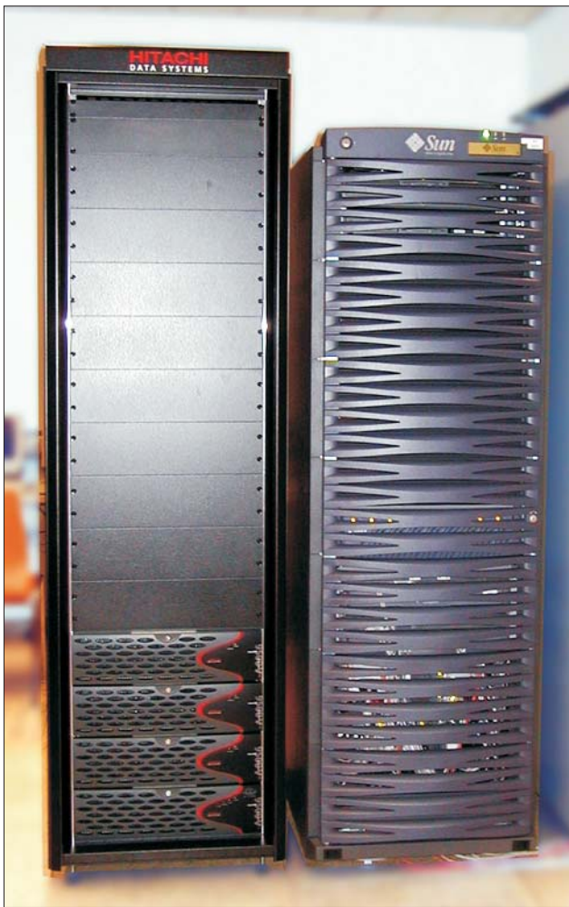
Hitachi Storage System, SWD Server SunFire 3800
